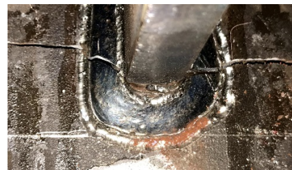
(b) Crack from HFMI groove on attachment
